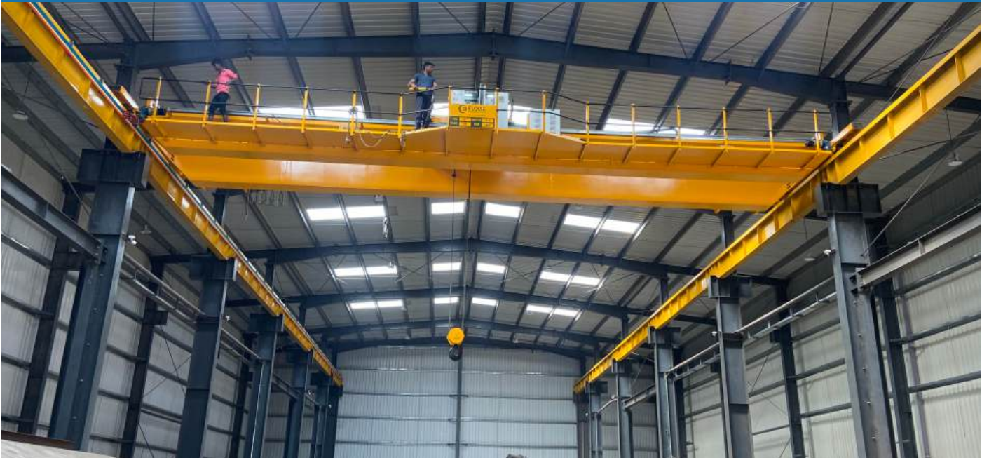
10 T DG EOT CRANE
